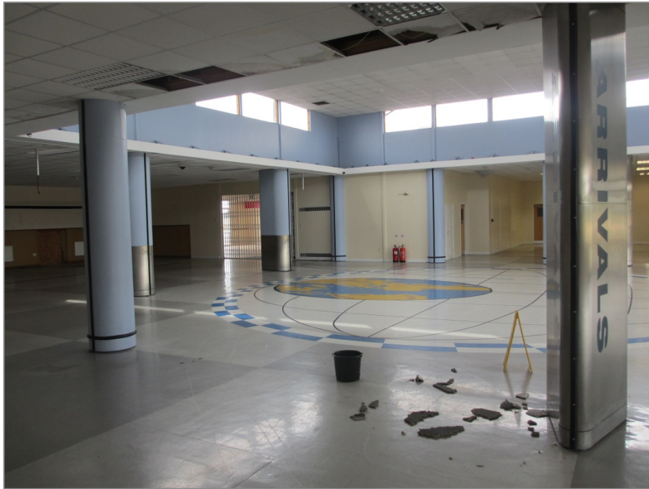
Figure 3: Main foyer of terminal building from arrivals. Check-in area to the left of the image.
