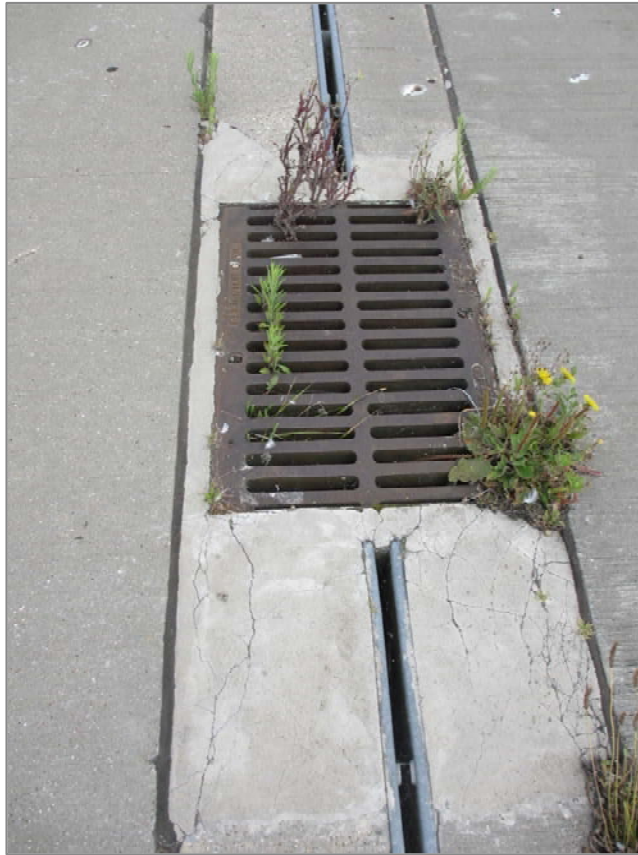
Figure 7: Apron Drainage. Some growth of plants which will need to be addressed.
